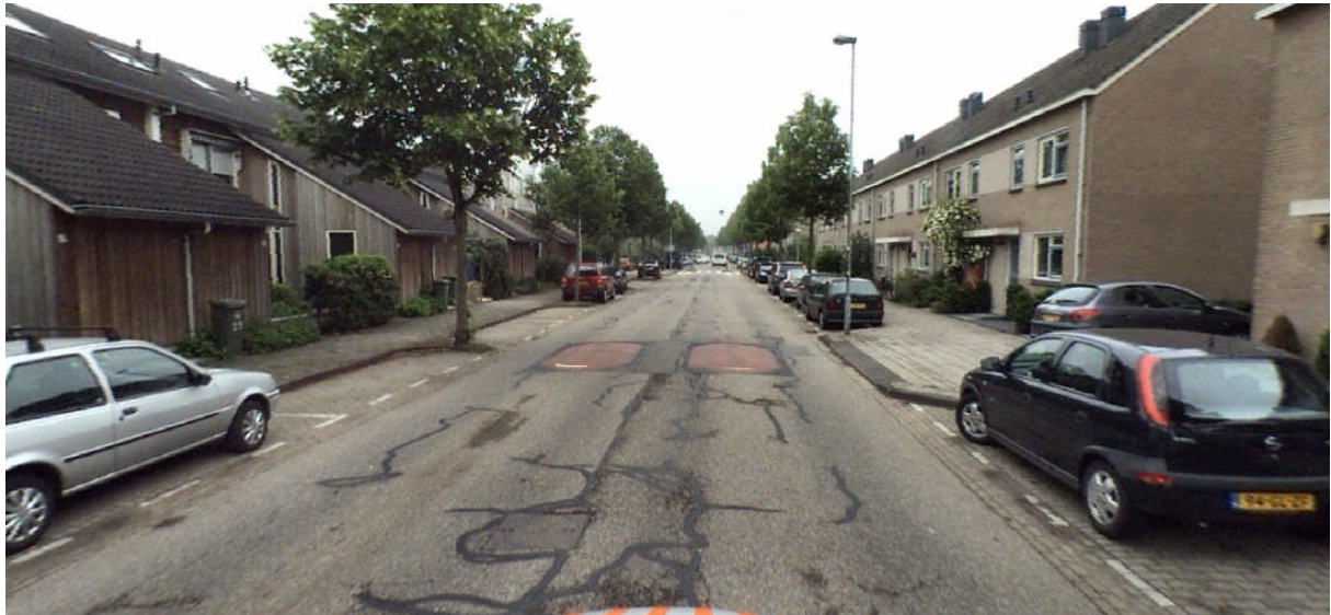
Foto 1: Amnesty Internationalweg: scheuren in asfalt
