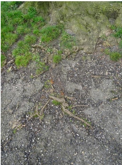
Links beworteling tot in de verharding,
